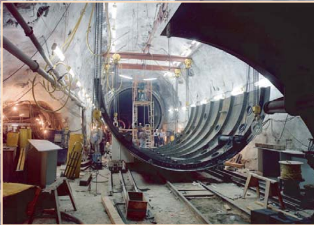
Line-of-sight pipes for tunnel experiment at Rainier Mesa, date unknown
