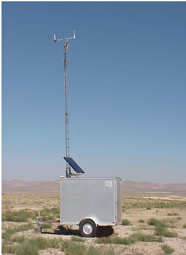
Figure 16-1. Example of a typical MEDA station with a 10-meter tower
