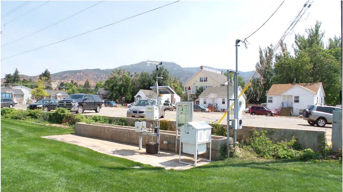
Figure 7-2. CEMP station in Cedar City, Utah
